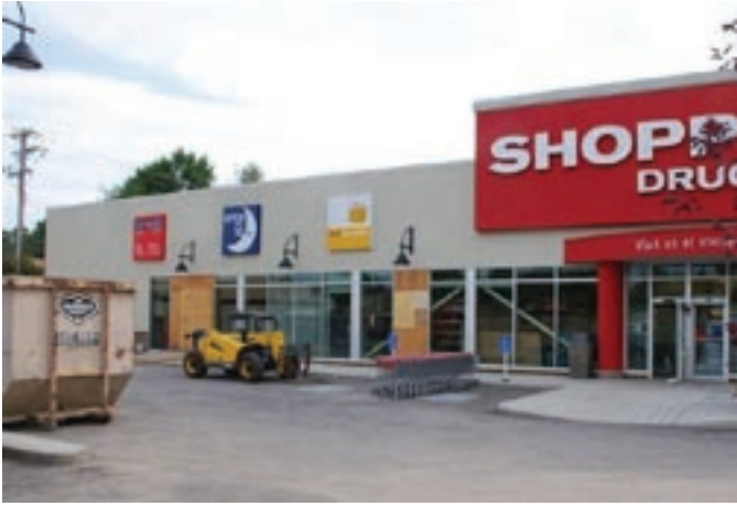
Figure 11 - Shoppers, 3 Avenue SE and Centre Street, August 15, 2013, flood damage.
